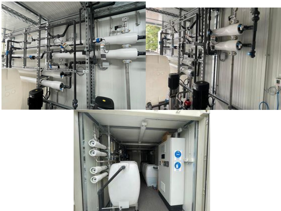
Figure 13. The NF and RO units
