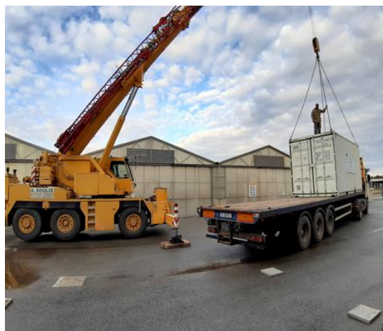
Figure 11. The NF, RO, MED, and Crystallizer installation in Larnaca
