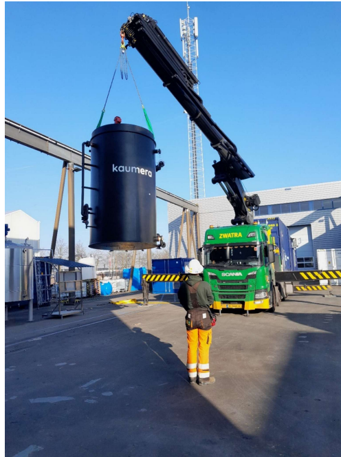
Figure 15: Transport of the cooling tank. On the left the swan neck and on the right the inlets for the cooling water are visible.
