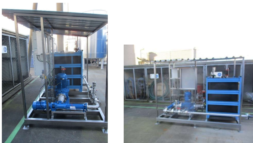
Figure 4.: The feed skid with a 1000 L feed buffer tank, a macerator and cavity pump.
