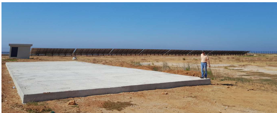
Figure 14: Concrete Slab for the pilot installation on site of the MWWTP Faro Olhão.
