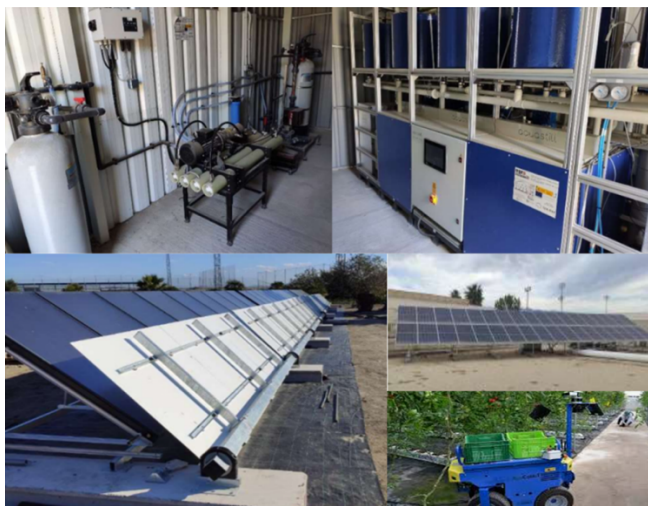
Figure 18. Desalination plants, sola energy fields and experimental greenhouse at CIESOL
